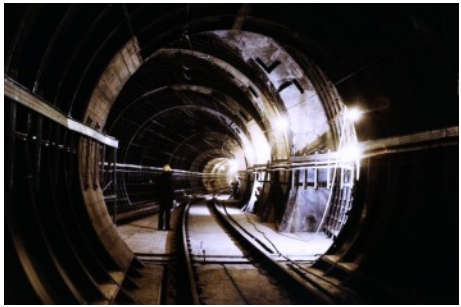
Figure 17 shows a sample chamber of a tunnel construction that is to be instrumented for a measurement programme.
